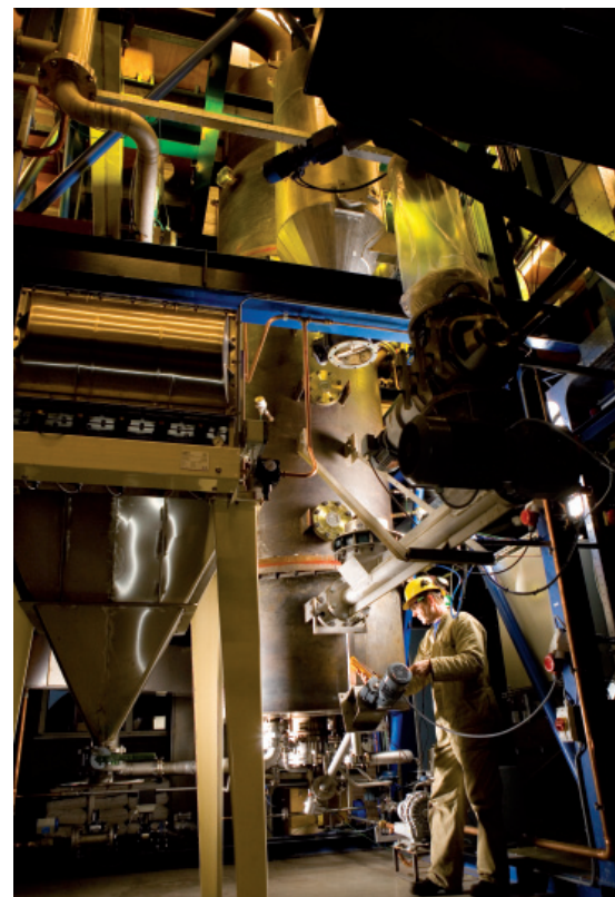
800 kW MILENA pilot gasifier
