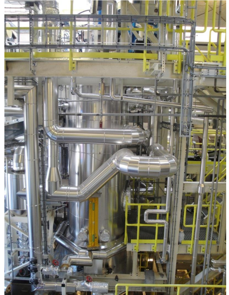
Torrefaction reactor process area
